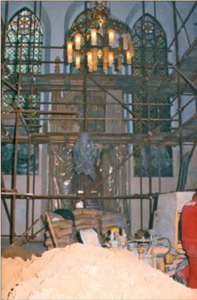
Repair and reconstruction of the interior of the Maisel Synagogue. As part of the building work, the heating system was repaired, tiles were renovated and the historic features of the interior (banisters, windows, gallery, etc.) were restored.
