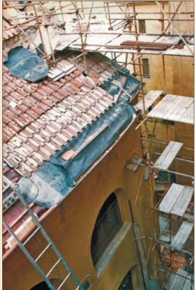
The repair and reconstruction of the Maisel Synagogue, which was undertaken in 1994-1995, began with the repair of the roof covering the nave.
